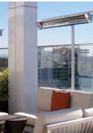
Hotel rooftop patio with custom W-Series pole mounted heaters
