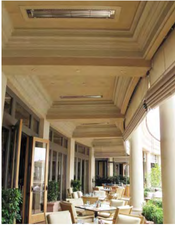
Luxury resort dining area with W-Series heaters flush mounted into a stucco coffered ceiling
